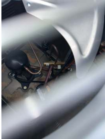
Photo of heat pump valve in a/c condenser outside.
