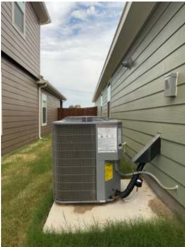
Not level Left Side Yard
