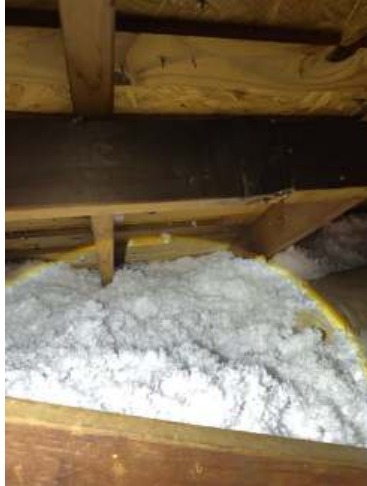
Blown in type of insulation.
