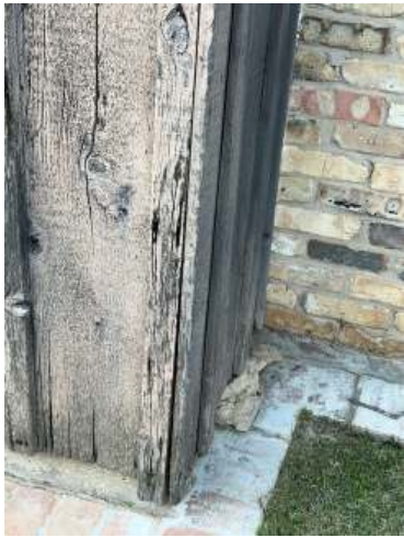
Wood trim deterioration.
