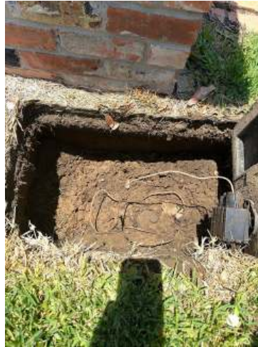
Water meter covered in dirt, this could cause premature failure. Recommend removing the accumulated dirt.
