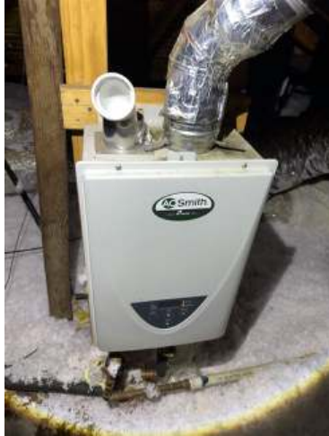
Instant hot water heater Attic
