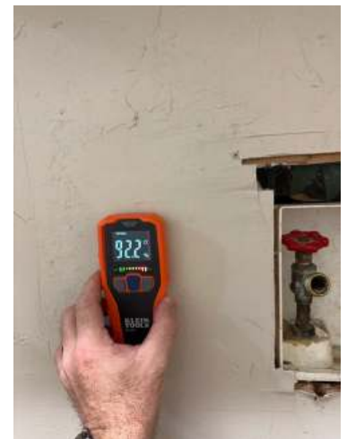
Moisture level found on the drywall in the laundry room near the leaking faucet.
