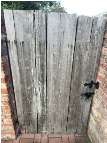
Wooden gate doors are deteriorating, recommend replacing the boards. Left, Entry, Side Yard
