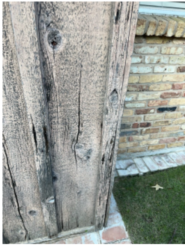
Wood siding deterioration as well as the trim work deteriorating.
