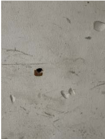
Multiple many holes like this throughout the garage. Recommend repairing to continue the fire rating in the garage. Garage
