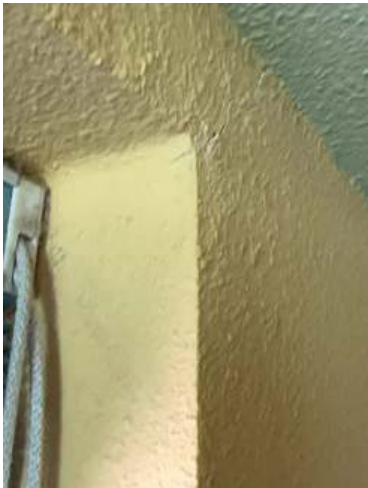
Drywall crack found above window in the primary bedroom adjacent to exterior brick crack on the exterior of the home. Primary Bedroom
