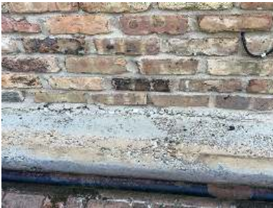
Exposed aggregate is visible along the exterior foundation wall. We recommend applying a concrete smoothing coat to protect the exposed rocks from water penetration and freeze-thaw damage. Rear
