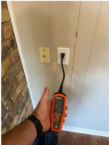
No power to the outlet, recommend electrician to evaluate and repair. Living Room
