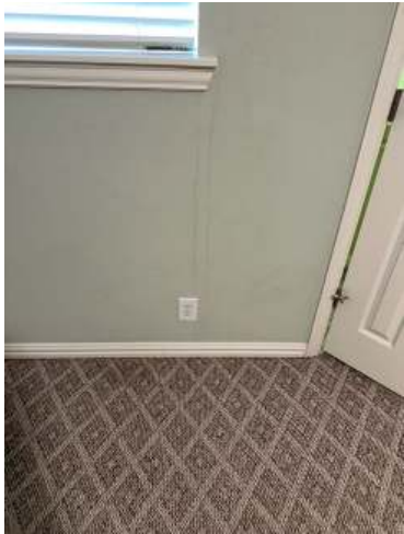
Water staining is visible on the interior wall directly below the window. We recommend having a qualified contractor evaluate this area to determine the source of the moisture and make any necessary repairs. Bedroom 3, Left
