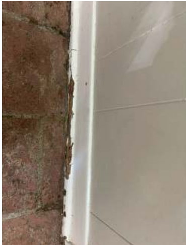
Wood trim deteriorated. Recommend repair. Eat in Kitchen
