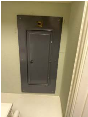
Main electrical panel. Bedroom 2, Bedroom Closet
