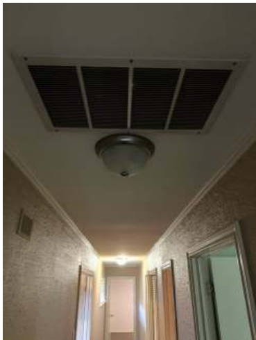
Bulb burnt out, replacement is recommended.
