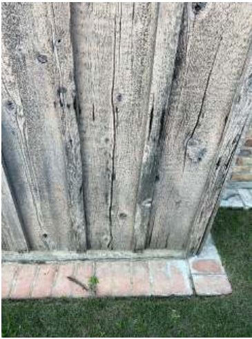
Wood siding deterioration.
