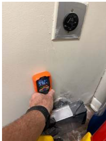
Moisture level found on the drywall in the laundry room near the leaking faucet.
