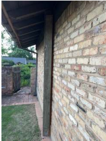
Unknown board spray foamed to the side of the house. Unknown reason for it to be there. Not structural.
