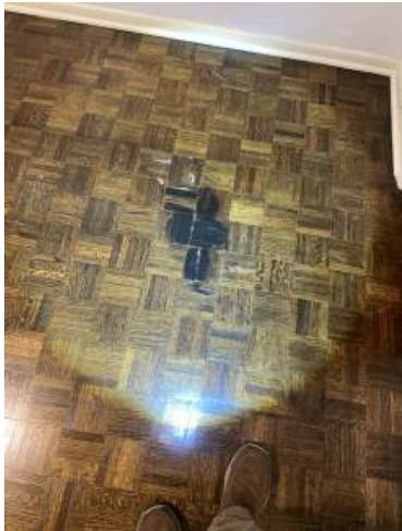
Floor damage. Bedroom 4
