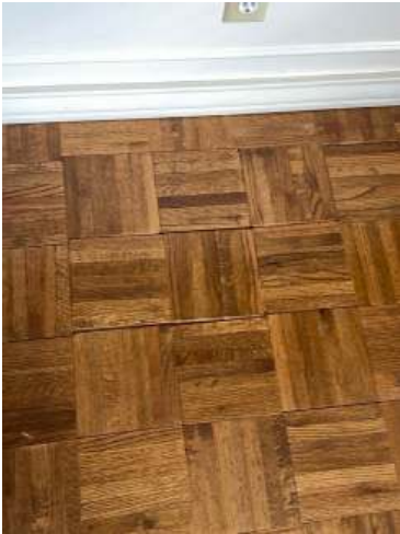
We observed loose flooring in the dining room. We recommend having a qualified contractor evaluate and repair this area. Dining Room
