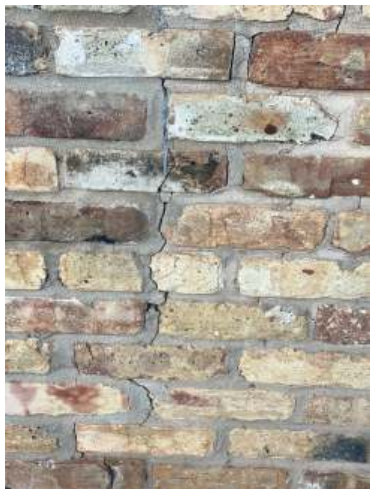
Crack found in the exterior brick on the left side of the home near the back. Continuing down through the foundation. Recommending evaluation by a structural engineer. Rear, Left, Side Yard
