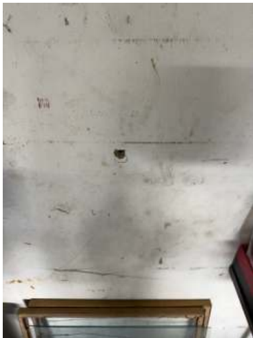
Multiple many holes like this throughout the garage. Recommend repairing to continue the fire rating in the garage.
