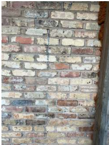
Attempt to add grout to the crack in the brick veneer, unsuccessful attempt. Left, Side Yard
