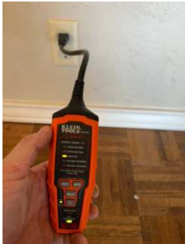
No power to the outlet, recommend electrician to evaluate and repair. Dining Room
