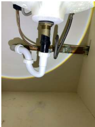
Tape wrapped around sink drain pipe in master bathroom.
