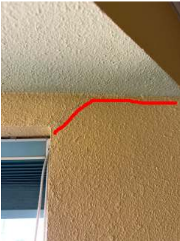
The line should help to find the crack in the drywall at this location. Recommend to monitor this area for any changes.
