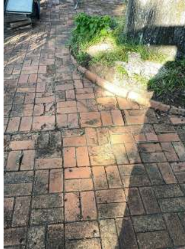
Tree roots lifting the brick pavers on the backyard side of the tree.
