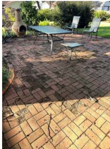
Patio bricks are spalling all over rear patio.
