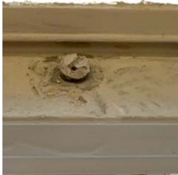
Example fo missing lock hardware on the window.
