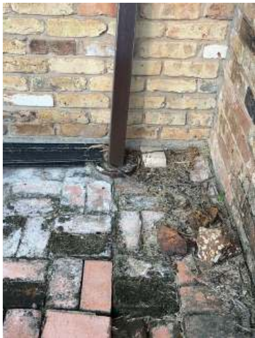
Downspout entering underground drainage pipe, unknown where the discharge is and whether or not the drainage pipe is blocked. Left, Side Yard
