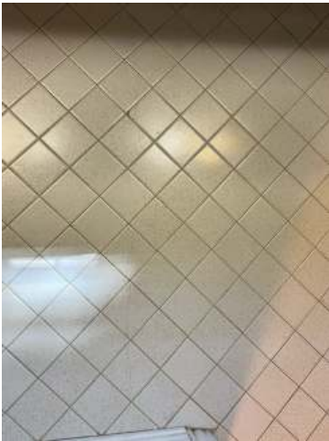
Jack and Jill Bathroom floor tile cracking Jack and Jill Bathroom
