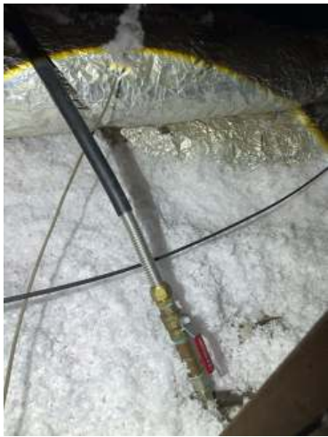
CSST plumbing found in the attic, recommend having an electrician verify a bonding wire is connected or having a bonding/grounding installed.
