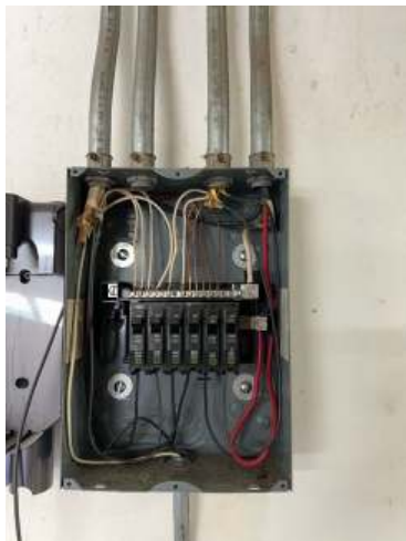
Inside look at the wiring in the subpanel.
