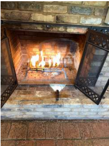
Perspective of gas fireplace operating as intended. Living Room
