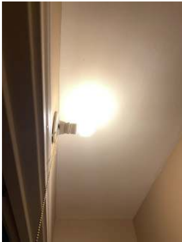
Protective cover recommended to protect light bulb from being damaged or broken. Hall Closet, Closet, Bedroom 2, Bedroom 3, Bedroom 4, Primary Bedroom
