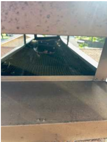
Spark arrester at the top of flue.
