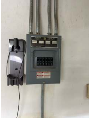
Sub panel in the garage.
