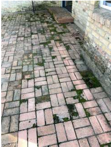
Moss growth on brick deck. Rear, Patio
