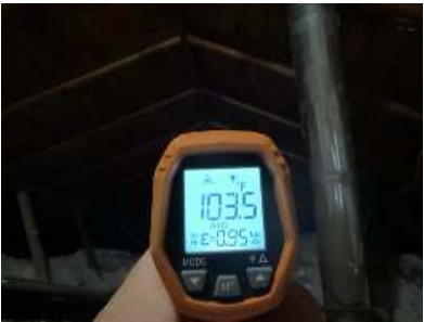
Temperature inside of attic space during the inspection.
