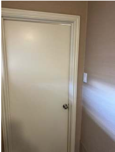
Large gap at the top of the latch side of the doo entering the front left bedroom, Bedroom 4. Bedroom 4
