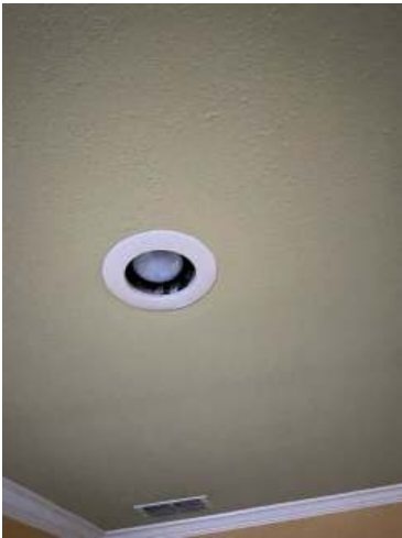
Possible bulb burnt out, recommend replacing. Primary Bedroom
