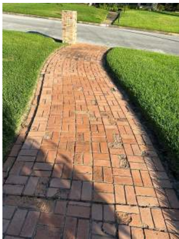
Brick pavers are spalling and settling down the entire path. Rebuilding the walkway base is recommended. Front Entrway
