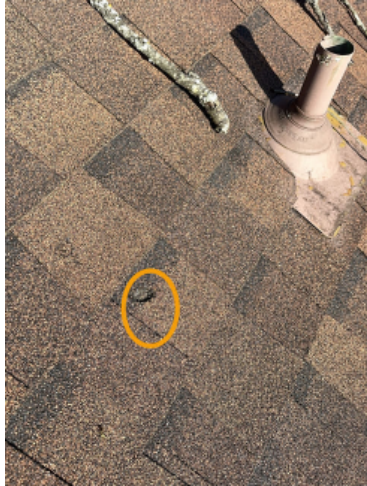
Damage to shingle, most likely from a fallen limb from the tree.
