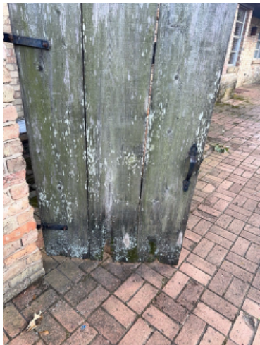
Wooden gate doors are deteriorating, recommend replacing the boards. Rear, Entry, Patio
