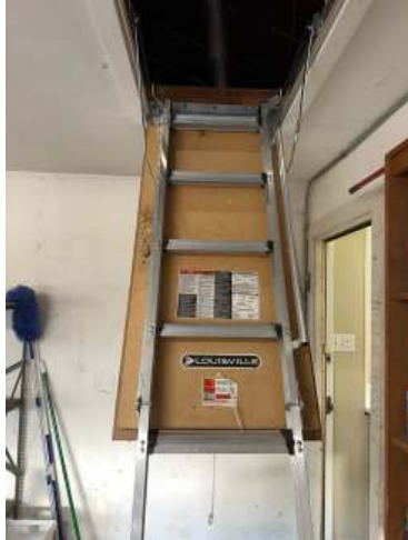
Attic ladder, not fire rated.
