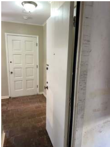
Recommend that self closing hinges be added to garage entry door. This was not available at the time this home was constructed, but has now been required by the IRC building code. Garage, Entry
