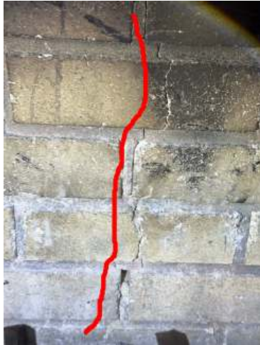
Crack in the fire brick and grout. This is an internal system and can be replaced by a fireplace contractor.
