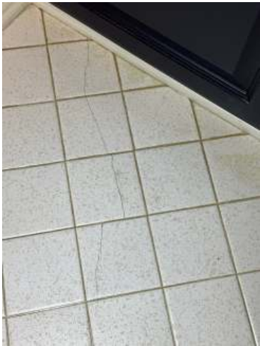
Cracked floor tiles observed in the Jack and Jill bathroom water closet. Recommend evaluation and repair by a qualified professional. Jack and Jill Bathroom
