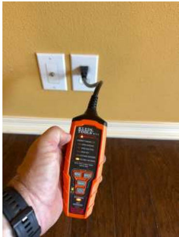
An outlet tester indicates a hot/neutral reverse wiring condition at the primary bedroom exterior wall facing the backyard. Repairs by a licensed electrician are recommended. Primary Bedroom
