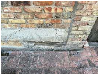
Exposed rebar Left, Rear
