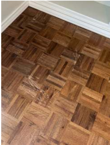
Dining room floor damage. Dining Room
