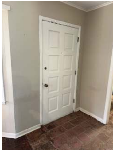
This rear exit door and the front door both need to be press closed in order to lock the deadbolt. Recommend the doors be adjusted so it is easier to lock them. Main Entry, Eat in Kitchen
