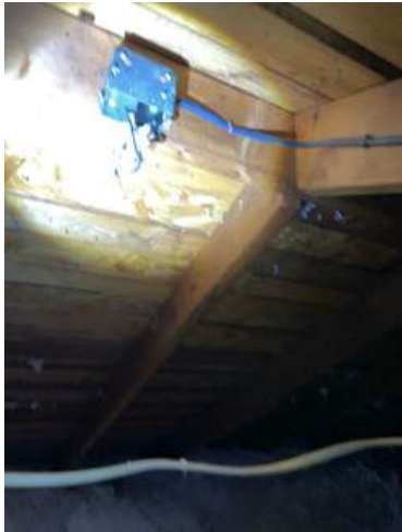
Electrical wires hanging out of a junction box in the attic with no wire caps, unknown if these wires are live. Attic
