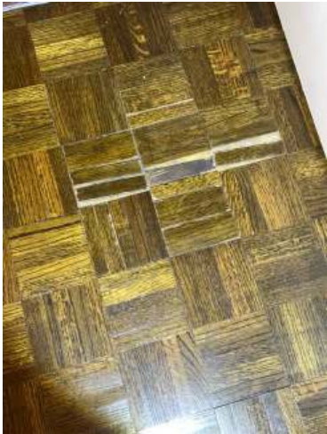
Floor damage in closet. Bedroom 4, Bedroom Closet
