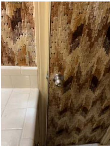
The door is rubbing at the latch. We recommend adjusting or modifying the door as needed for proper operation.
