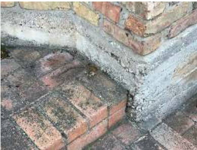
LineItem: A. Foundations". Image shows foundation corner with brick steps. I described "exterior foundation corner where we observed some exposed aggregate in the concrete." This is factual, visible, and directly Rear
