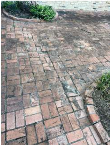
Brick pavers are spalling and settling down the entire path. Rebuilding the walkway base is recommended.
