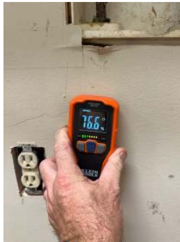
Moisture level found on the drywall in the laundry room below the leaking faucet.
