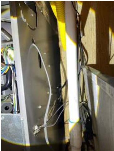
Here we can see a missing or displaced bushing where the wire enters the heating equipment cabinet. This can lead to wire abrasion over time. We recommend having a licensed electrician evaluate and install a Hallway, HVAC
