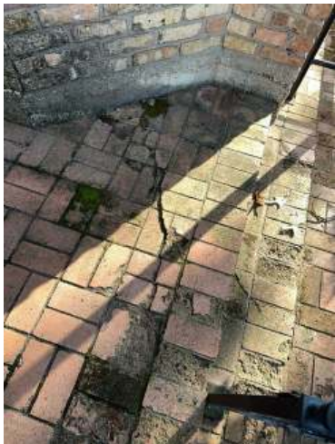
Minor settling of the rear porch at rear left side of the home. Recommend monitoring for activity. Back Yard, Patio
