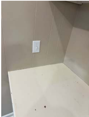
Unknown if this switch is working for the built in desk in the living room. there are lights under the cabinets above that could not be turned on. Living Room
