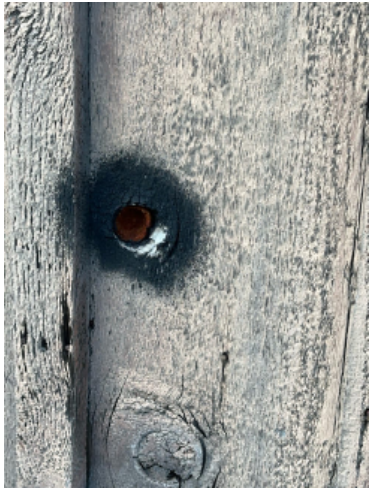
Another entry point into the house that needs to be sealed.
