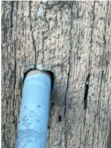
Gas line entering the house. Recommend caulking this entry point to stop moisture and insects from entry into the home. Left, Side Yard
