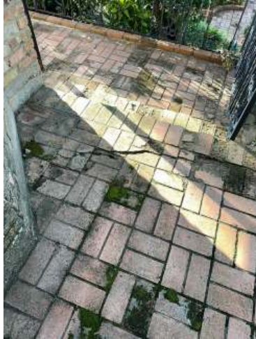
Settling crack in patio.
