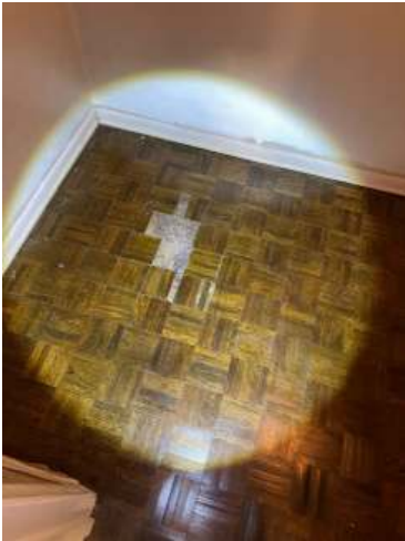
Floor damage in closet. Bedroom 4, Bedroom Closet
