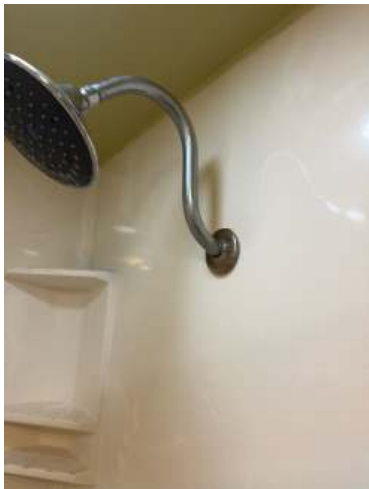
Shower head loose in the wall. Not leaking.
